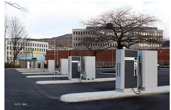
City ring charge hub in Norway: 10 (!) DC fast chargers on 1 site
